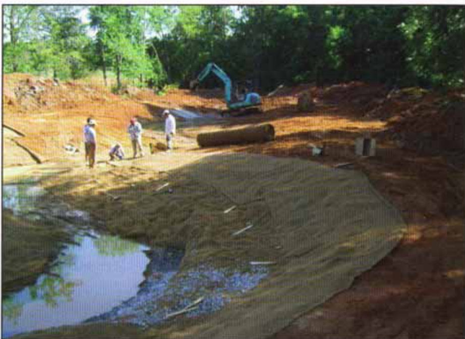
One type of woven coir erosion control blanket, designed to protect soil from higher flow velocities, was installed in the stream channel. A coir blanket with a more open weave was placed higher up the stream banks where stream flows are likely to be slower.
